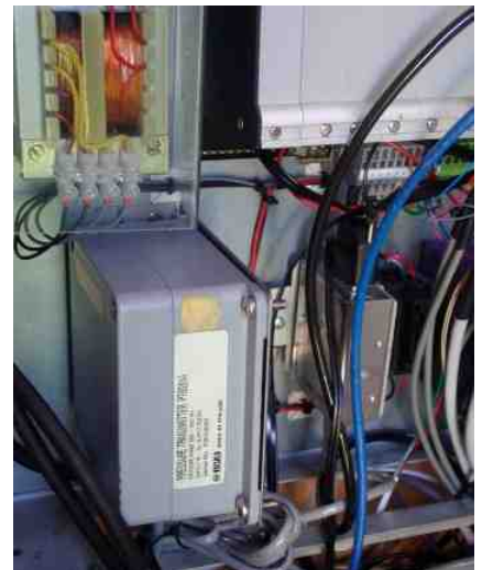
An air pressure sensor (Vaisala PTB pressure transmitter) installed inside a weather-station enclosure at a Finnish Meteorological Institute site. Temperature-compensated pressure and sea-level pressure measurements are calculated by the logger.
